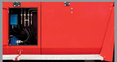
Pressurized Hydraulic Oil tank
